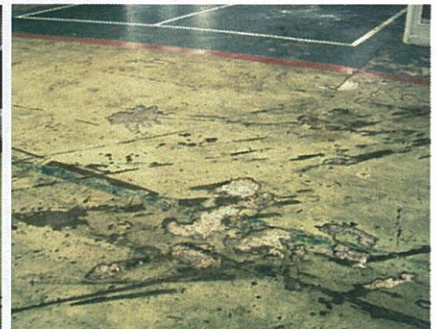
PU floor failure due to wear and tear at a basement car park
