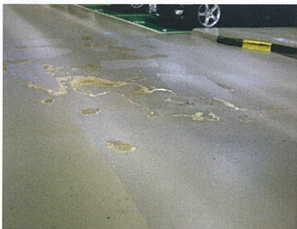
PU floor fails under heavy traffic near car park entrance.
