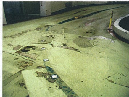
PU floor failure requiring extensive and frequent repairs
